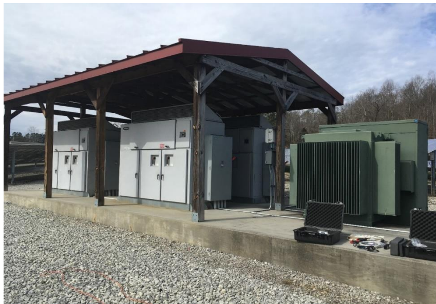
Four DC-AC Inverters 8.4kV Transformer
